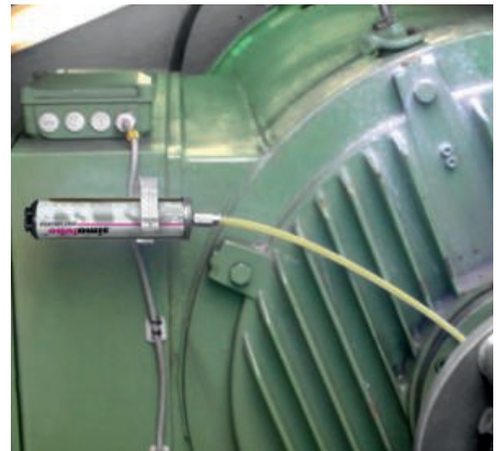
With the simalube 250ml lubricator, the generator is continuously supplied with lubricant for up to 12 months.
